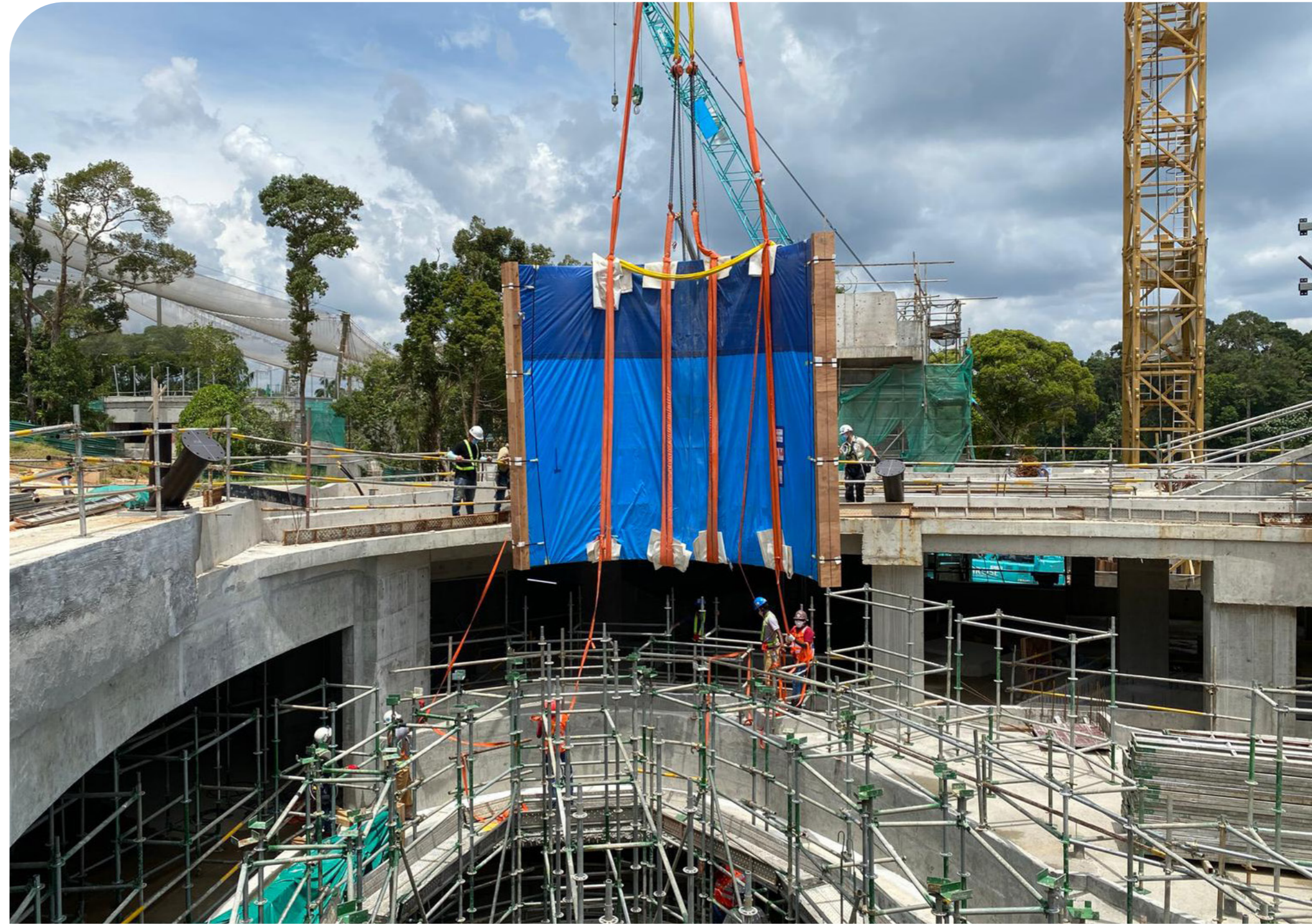
ABOVE: Installation of one of the acrylic sheets at Penguin Cove in the new bird park.
