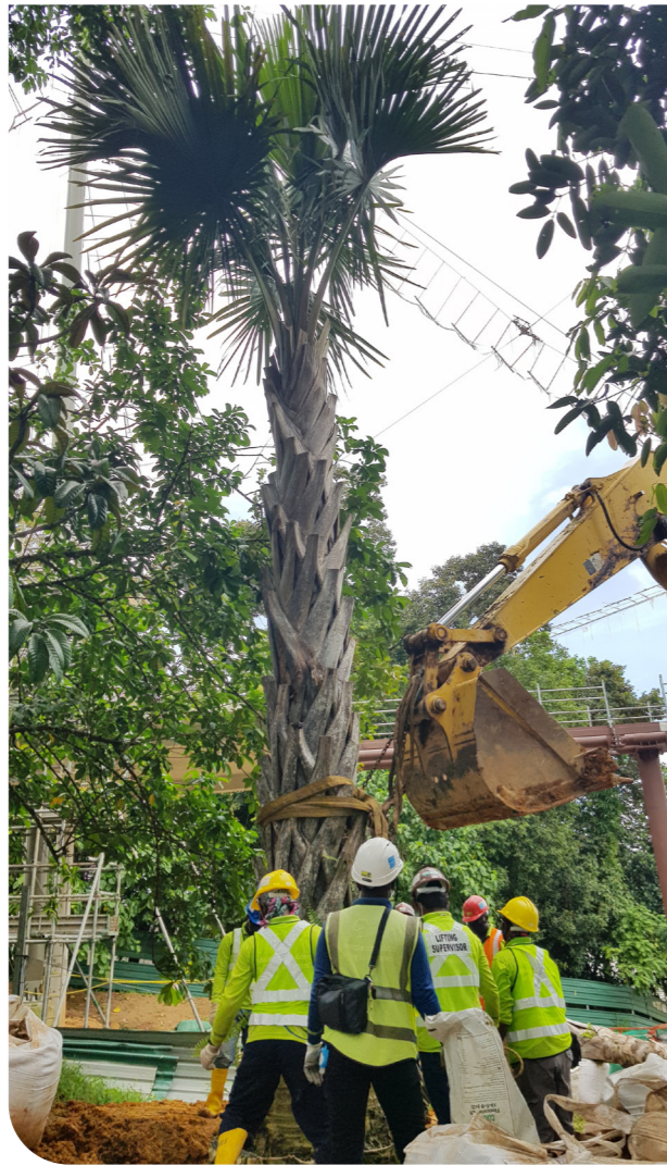
ABOVE: At 12m tall with a girth of 2.7m, this tailpot palm is the largest palm to be planted in the new Bird Park.
