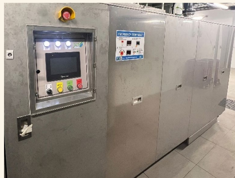
An onsite food waste digester.
