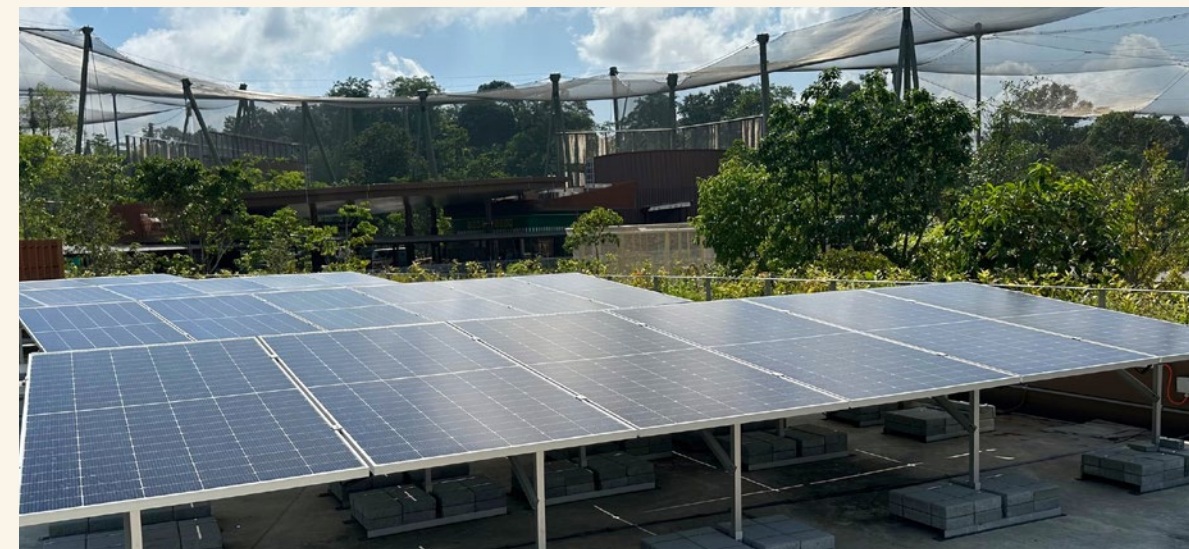
Solar panels installed across Mandai Wildlife Reserve harness clean energy, supporting sustainable operations.
